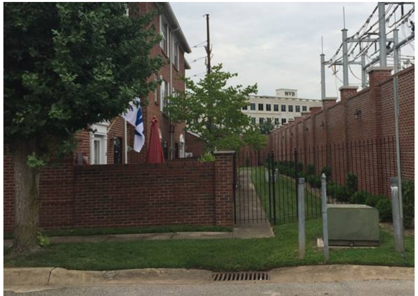
Figure 3 (bottom): The substation as built, demonstrating the fidelity of the final product to the design in Figure 2, above.
