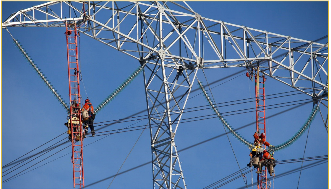
Crews string cable that stretches more than 500 km along the route of the Fort McMurray West 500-kV Transmission Project
