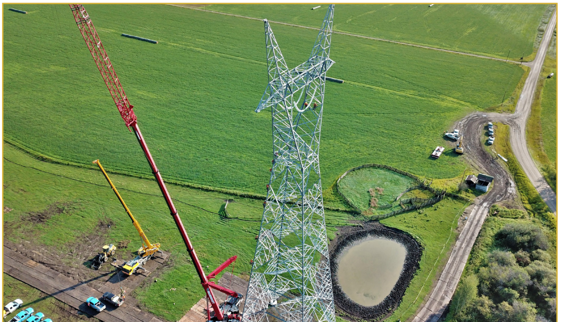
More than 1,350 transmission towers make up the Fort McMurray West 500-kV Transmission Project
